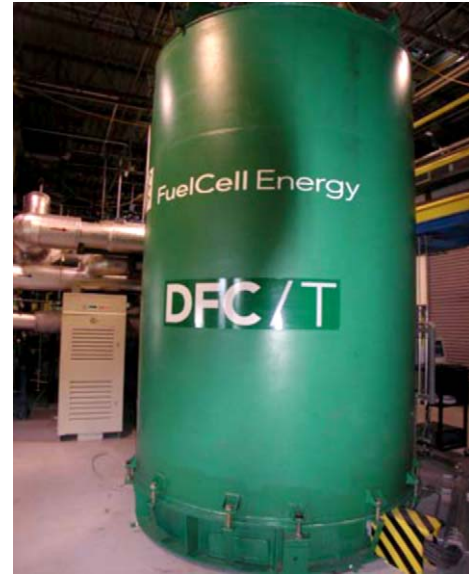
Fig. 2. Sub-MW DFC/T hybrid power plant facility: full-size DFC stack was integrated with capstone C60 micro-turbine.
